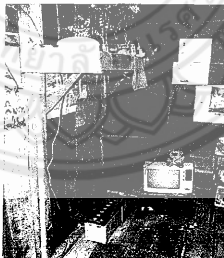
Figure 19 Inappropriate locations of battery and poor wiring.
