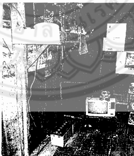
Figure 19 Inappropriate locations of battery and poor wiring.
