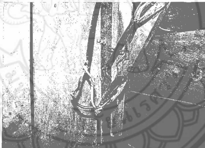
Figure 20 Poor wiring connections without insulation in a house at Ban Pean Village
