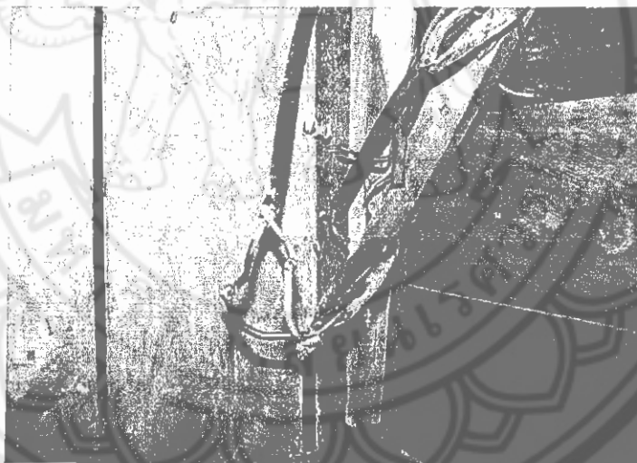
Figure 20 Poor wiring connections without insulation in a house at Ban Pean Village
