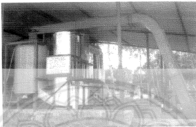
Figure 13 Gasifier system installed in Maharashtra, India
