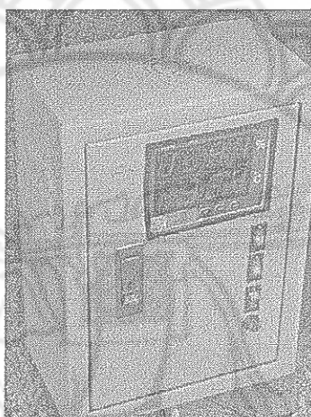
Figure 20 Control Panel of an Automatic Ignition System
