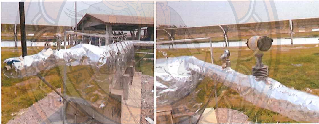
Figure 22 Thermal Energy Storage Prototype with insulation
