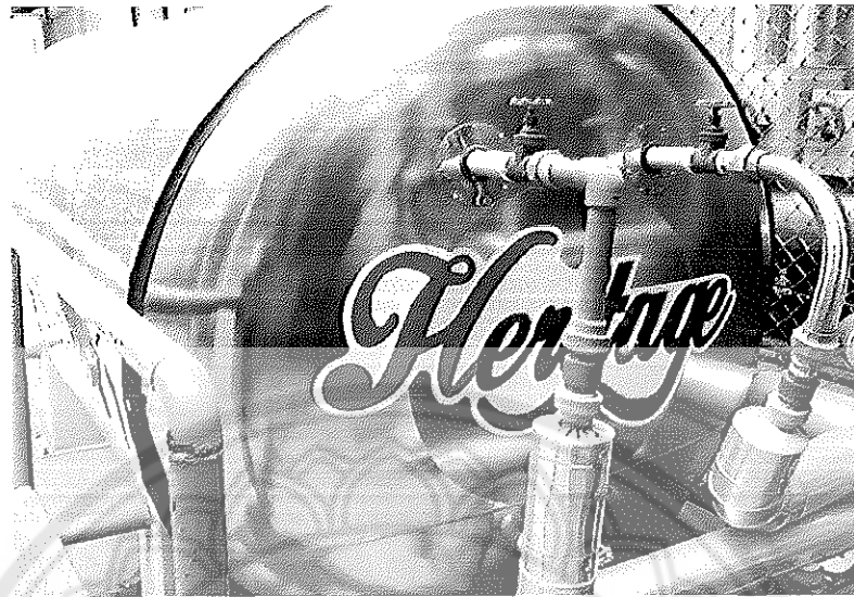
Figure 18 Hot Water Tank
