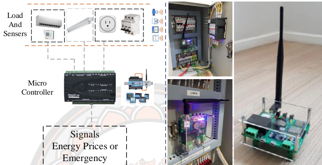
Figure 34 An example of the control system (hardware) of the aBEMS-IoT
