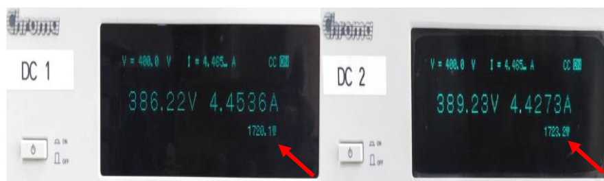
Figure 42 The total power of PV Simulator
